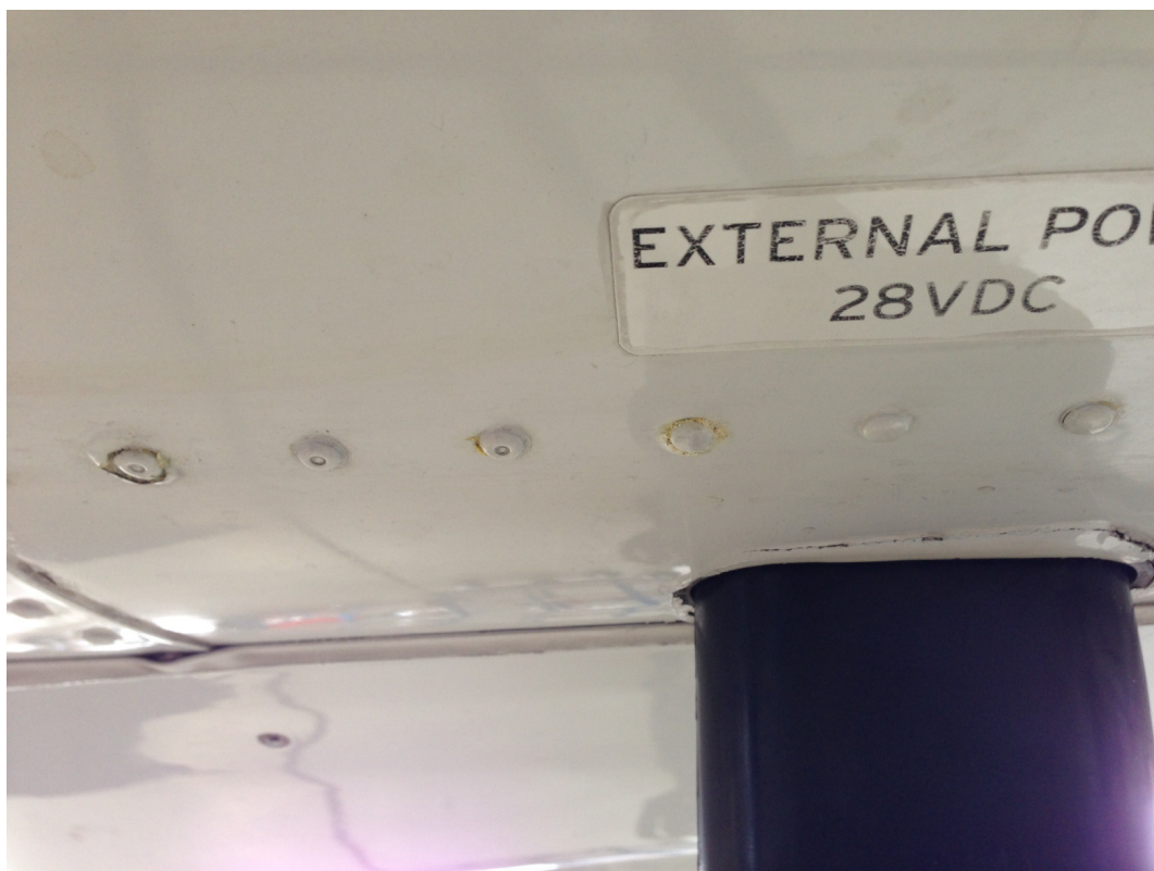
Figure 2. External Power Receptacle Rivet Corrosion
