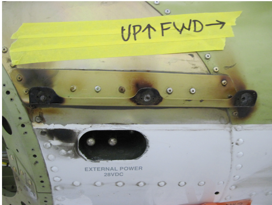
Figure 1. Electrical Damage Example
