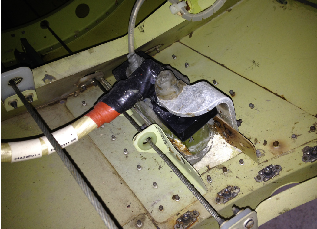
Figure 5. Internal Electrical Damage
